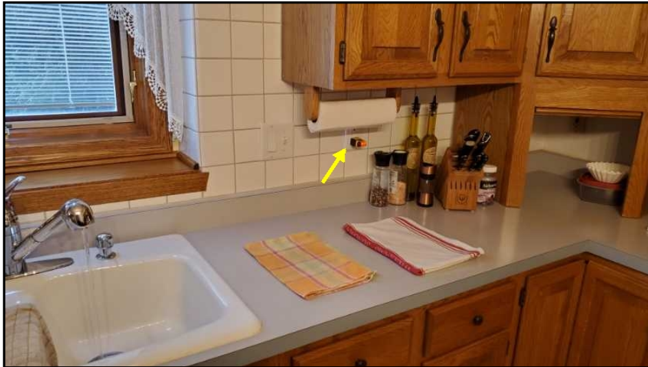
Failed GFCI testing
