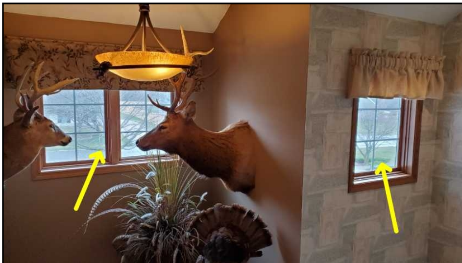
Failed double pane windows
