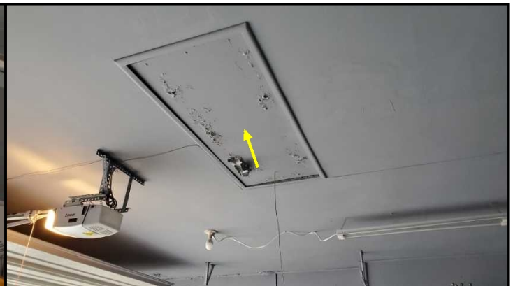
Fire barrier between garage and house broken
