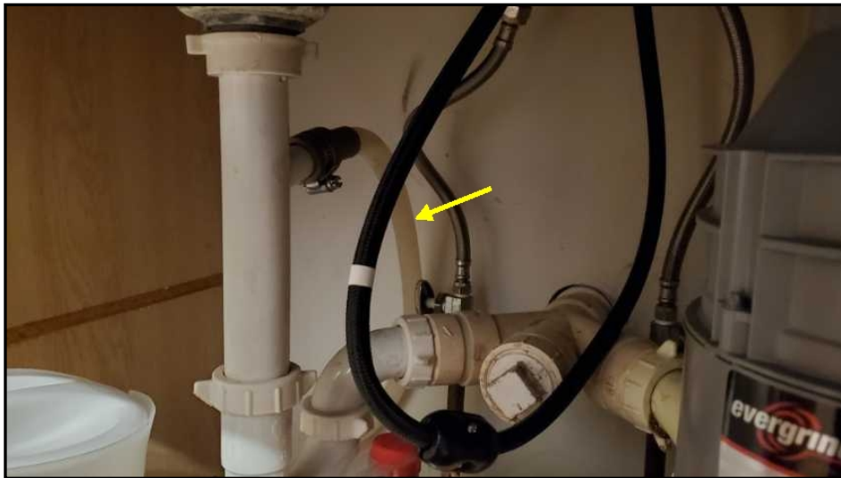
Dishwasher drain line no air gap device
