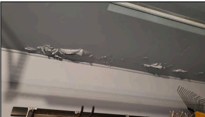
Peeling paint on ceiling
