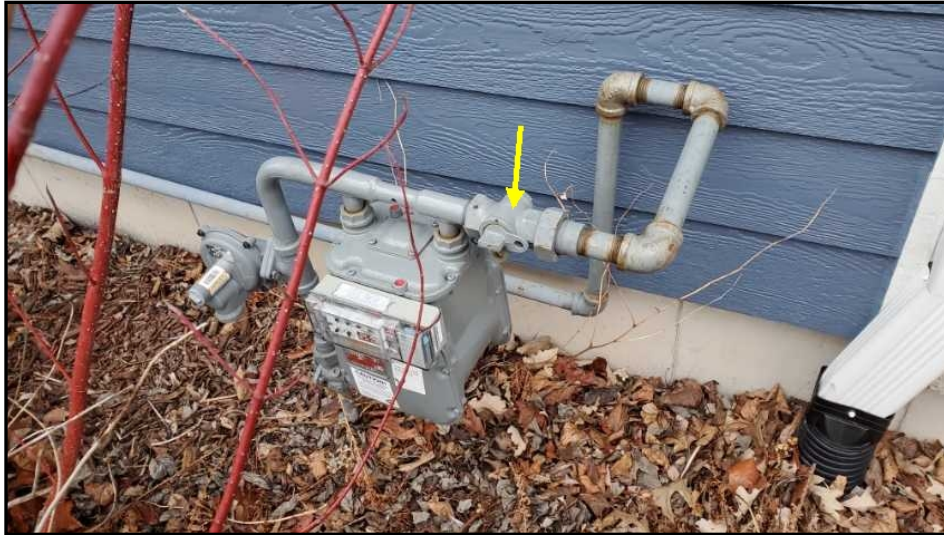
Main gas shutoff valve
