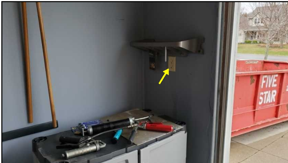
Failed GFCI testing
