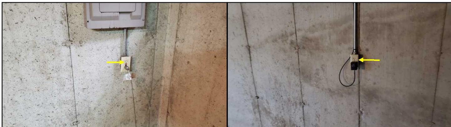
Failed GFCI testing
