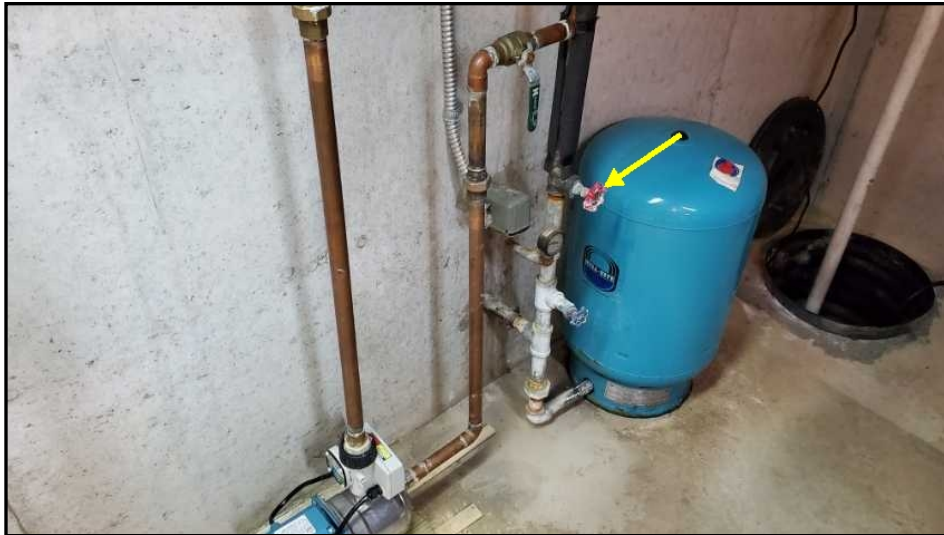
Main water shutoff valve
