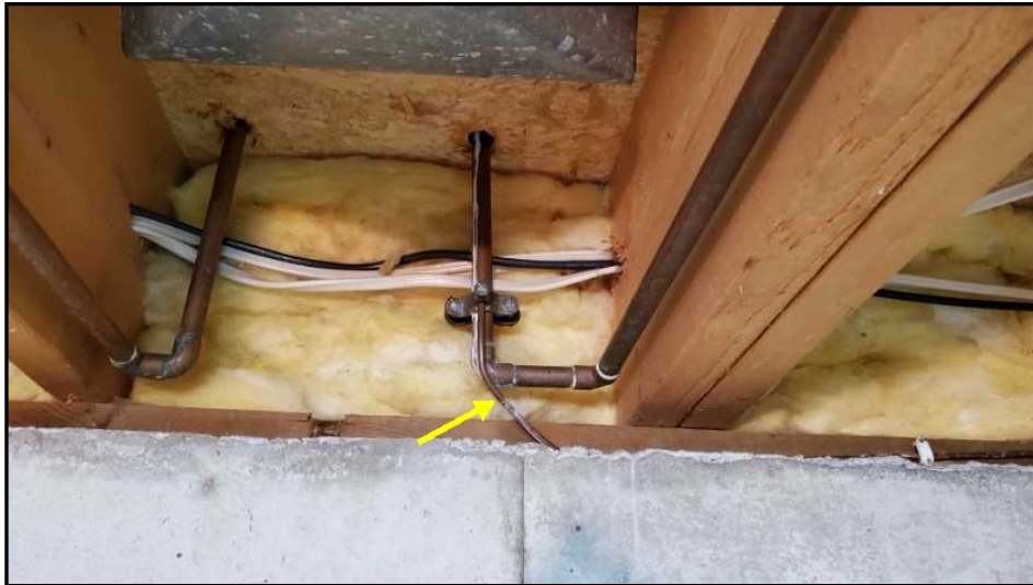
Ground to water pipe
